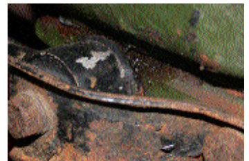
Slight bubbling from join is just visible
